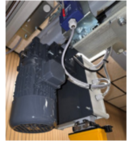
Motorized bridge and limit switch
